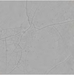
Cracked grey 20MM
